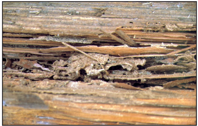
Figure 11. Damage in wood.
