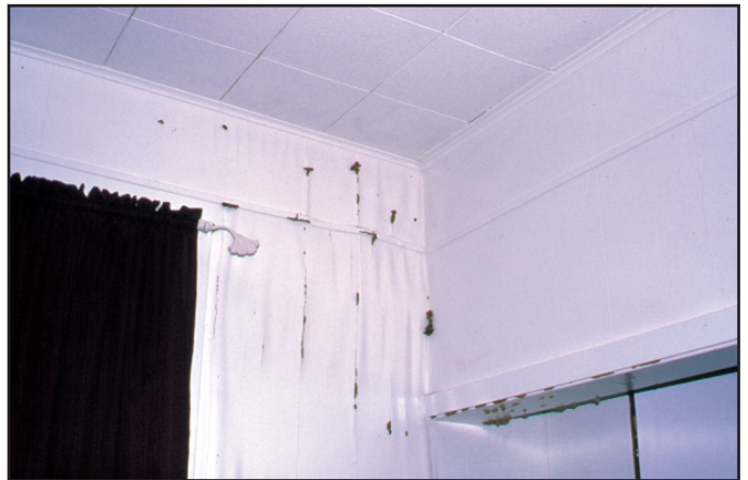
Figure 13. Shelter tubes on interior walls.
